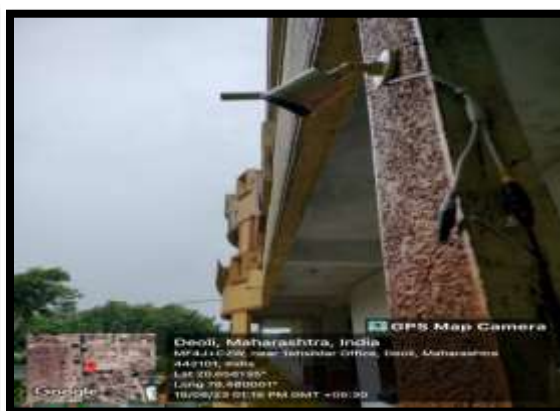
CCTV camera in front
